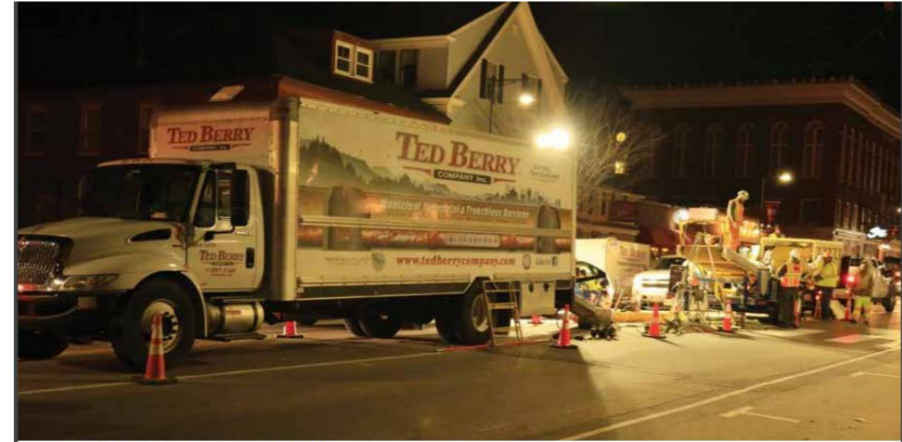
Each segment could be installed without bypass pumping if the work was done at night
