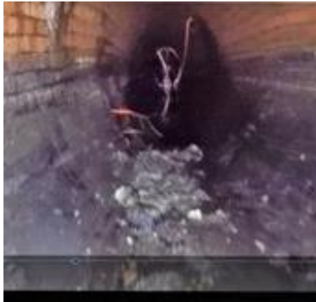
Suffering from mortar failure and infiltration.
