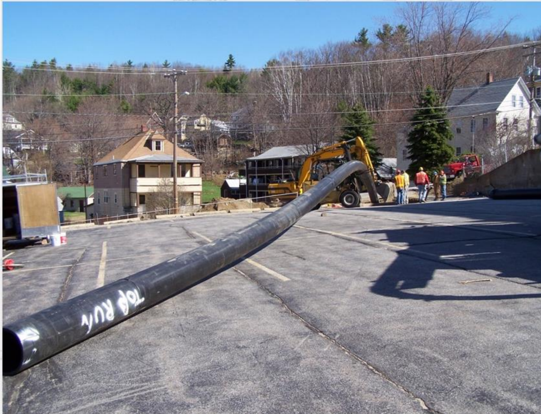
CONTINUOUS ( Can be HDPE or PVC) Slip Lining 24" CMP storm culvert with new 21" HDPE pipe
