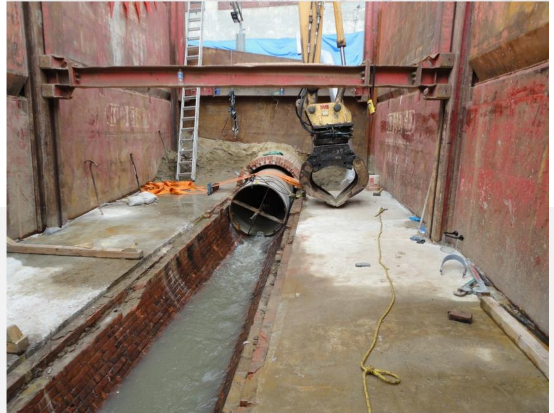
SEGMENTAL (Various Materials Available) Slip Lining 48" brick combined sanitary sewer with new 42" Hobas Pipe
