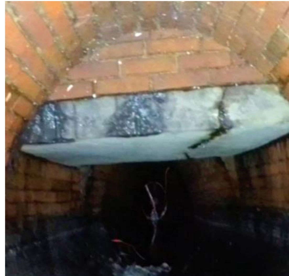
Three concrete beam "obstructions" inside sewer prevented CIPP lining.
