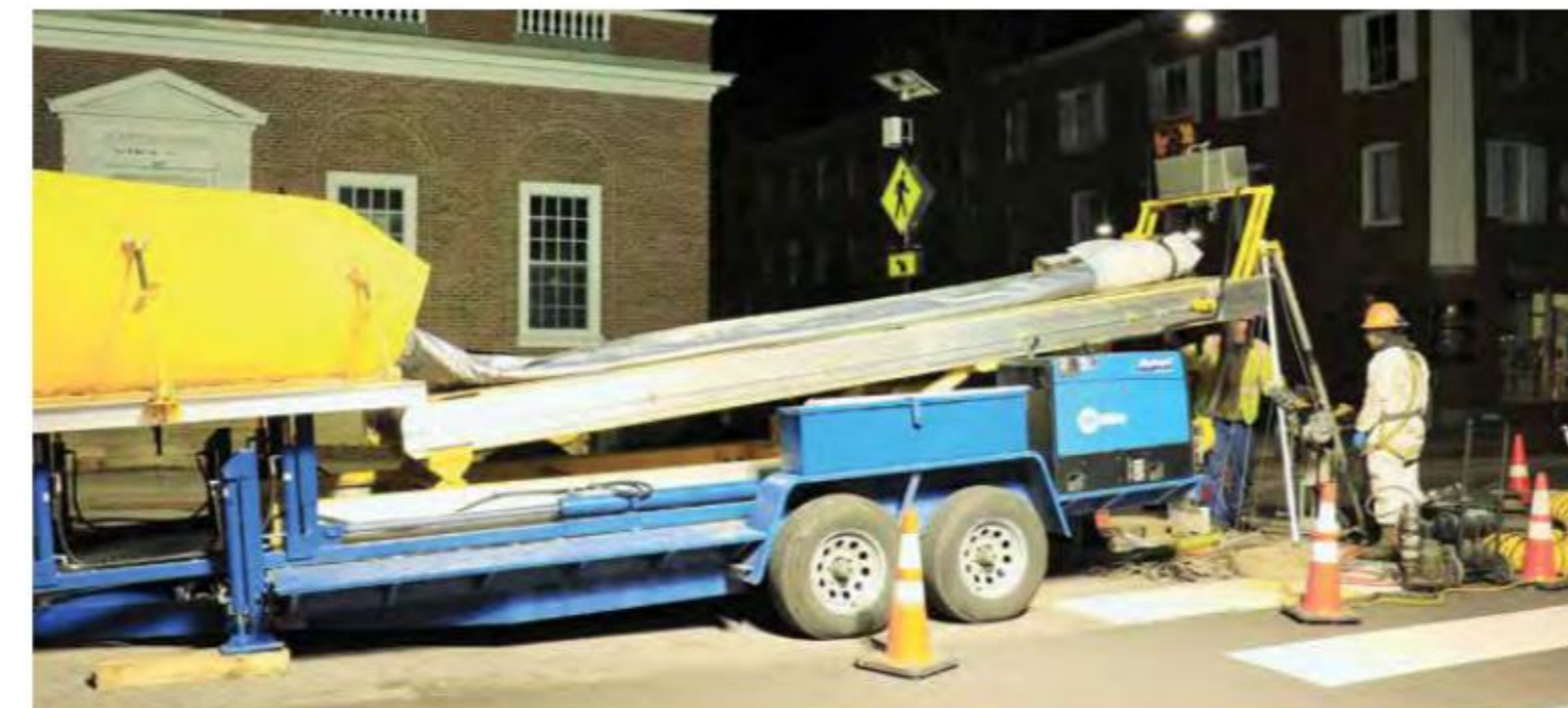
A motorized conveyor load system was used for liner placement into the existing manholes
